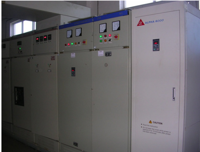
FIG. Inverter under Operation
